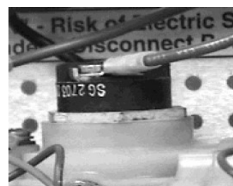
Figure 11: Installed heating element
